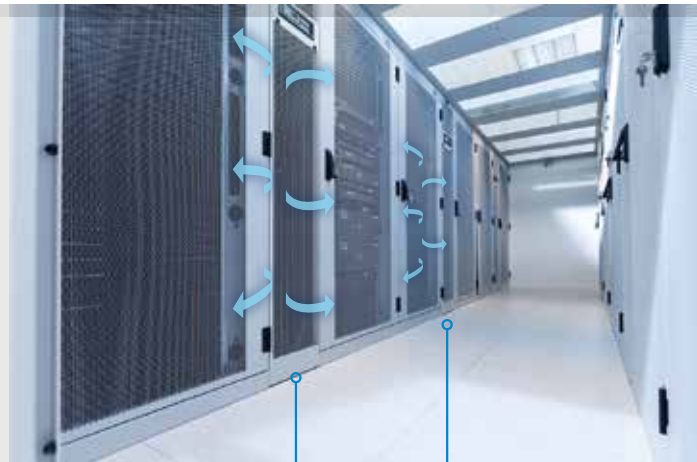
Example of H2O in Cold Corridor
