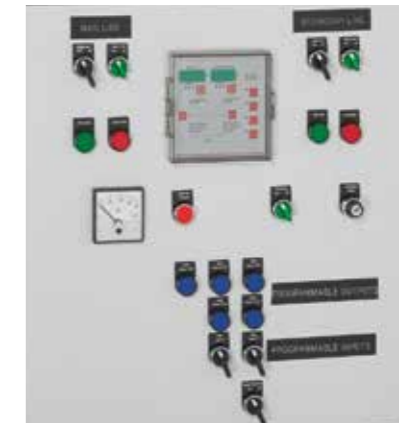
Control panel of a supply inverter with automation control unit Cat. N° 261 93
