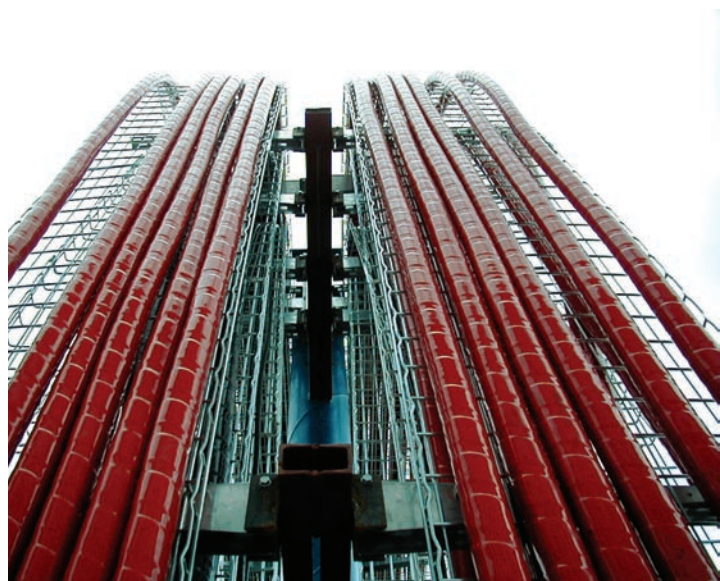
Example of more space busy by cable tray distribution
