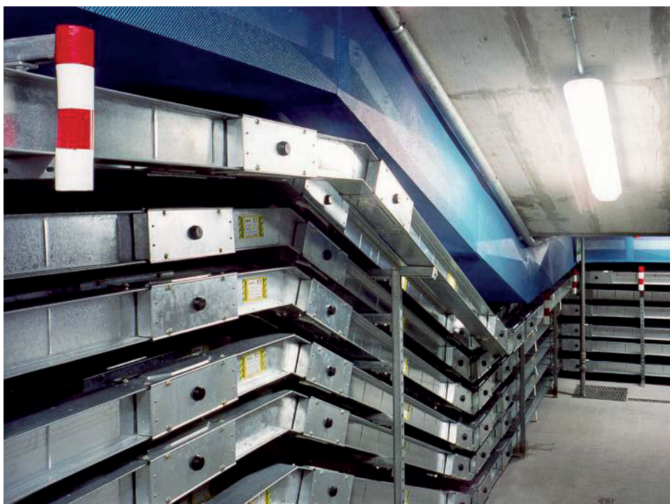
Example of high power distribution
