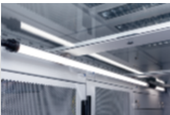
1 LED lighting → SEE P. 65
