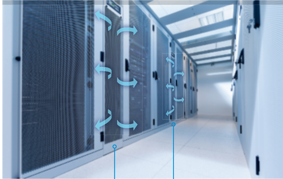
Example of H 2 O cooling system in cold aisle containment
